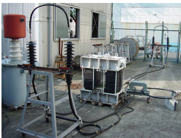
Fig. 4.3 Test situation of long-term outdoor power supply
