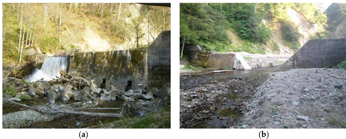
Figure 2. The check dam before (a) and after (b) the partial dam removal implemented in February 2009.
